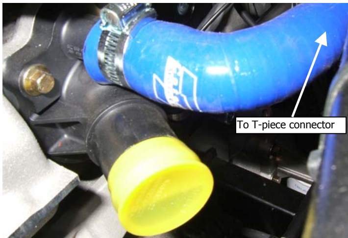
Figure 28 – Water circuit plumbing (water pump)
